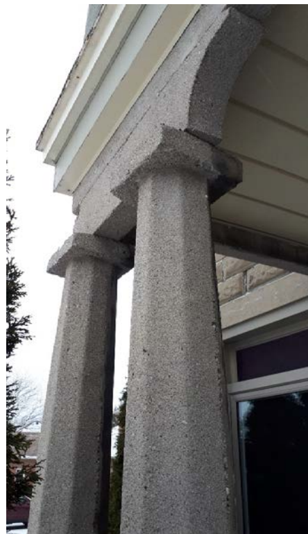
A closer view of concrete columns with a simple square capitals and entablature. Pre-war concrete porches are fairly rare features and likely the only ones existing in the municipality (Parsons, 2019).
