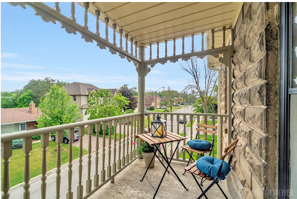
Showing the condition of the porch's upper balcony, facing north (Trentadue Torres Group, 2019).
