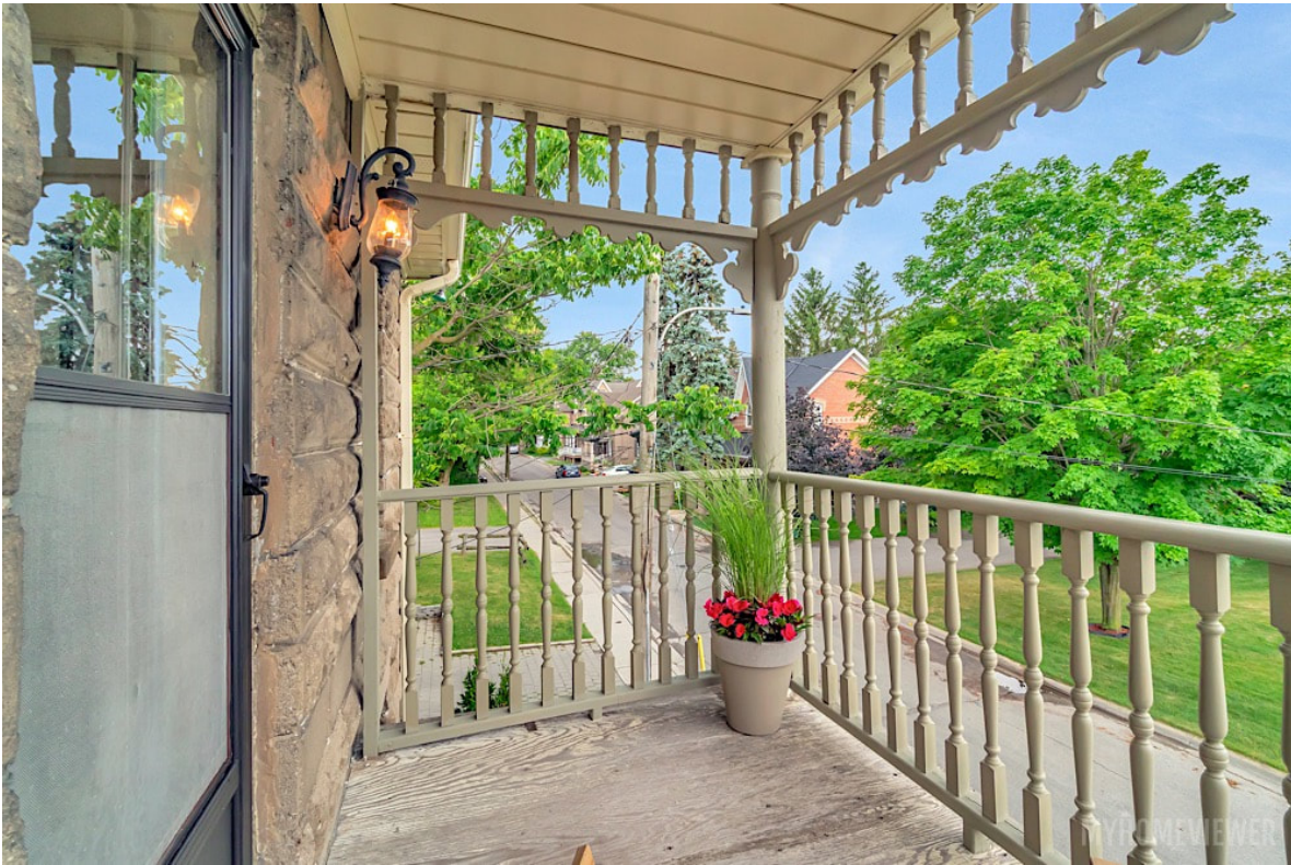
Showing the condition of the porch's upper balcony. The decorative wood trim and balustrade accents, although not original features, provide a complimentary accent to the standardized rusticated concrete cladding (Trentadue Torres Group, 2019).
