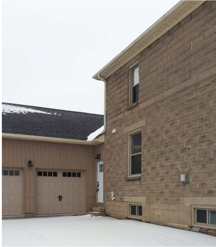
A closer view of the north wall and attached garage addition (Parsons, 2019)
